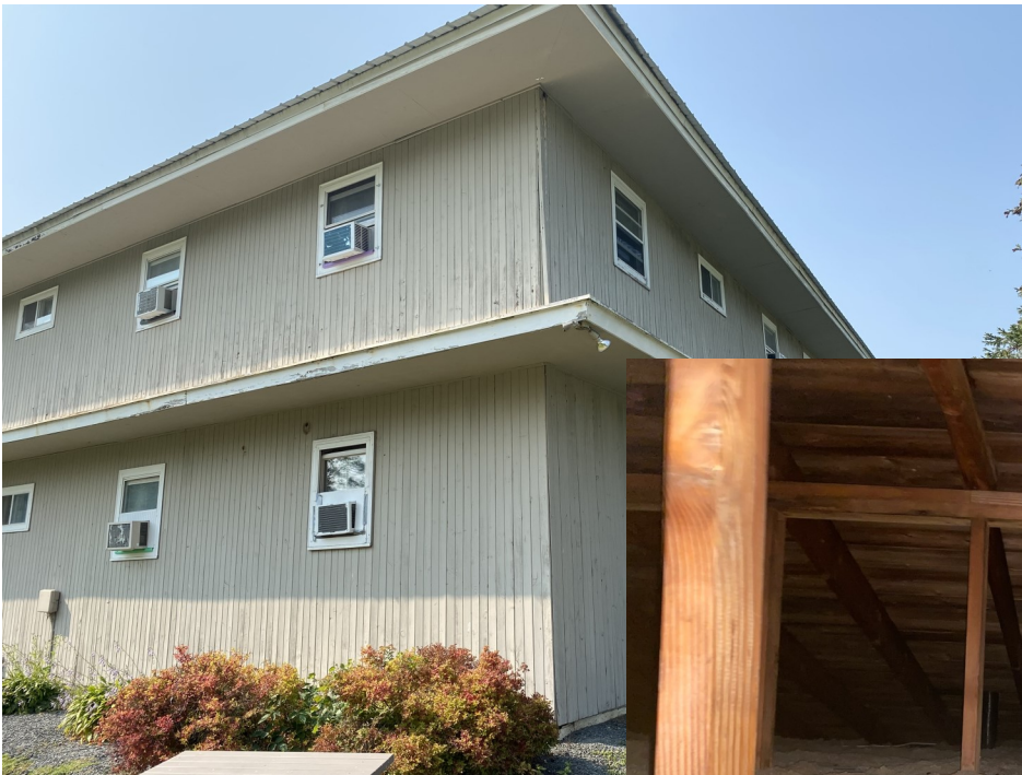
(left and below) Currently has non-breathable soffit 2nd floor and no air chutes in attic space
